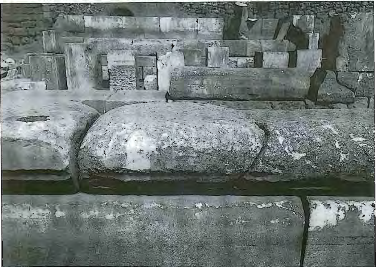
Pl.1-60 Deterioration of a stylobate block on the front
