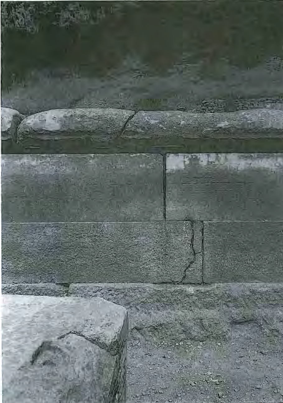
Pl.1-58 Breaking off of a block on the north wall
