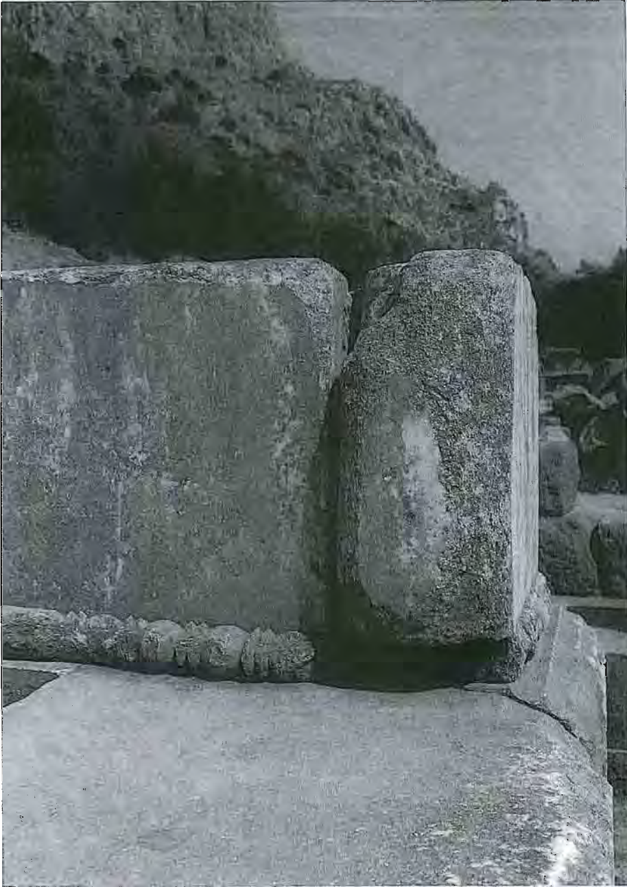
Pl.1-61 Deterioration of an orthostate block on the east anta
