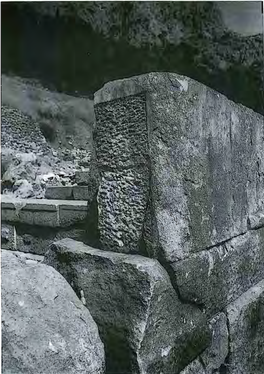
Pl.1-63 Deterioration of an orthostate block on the cross wall
