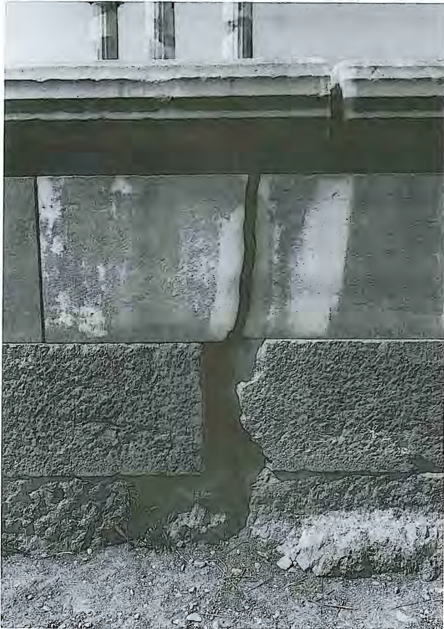
Pl.1-56 Crack and dislocation of blocks on the east wall
