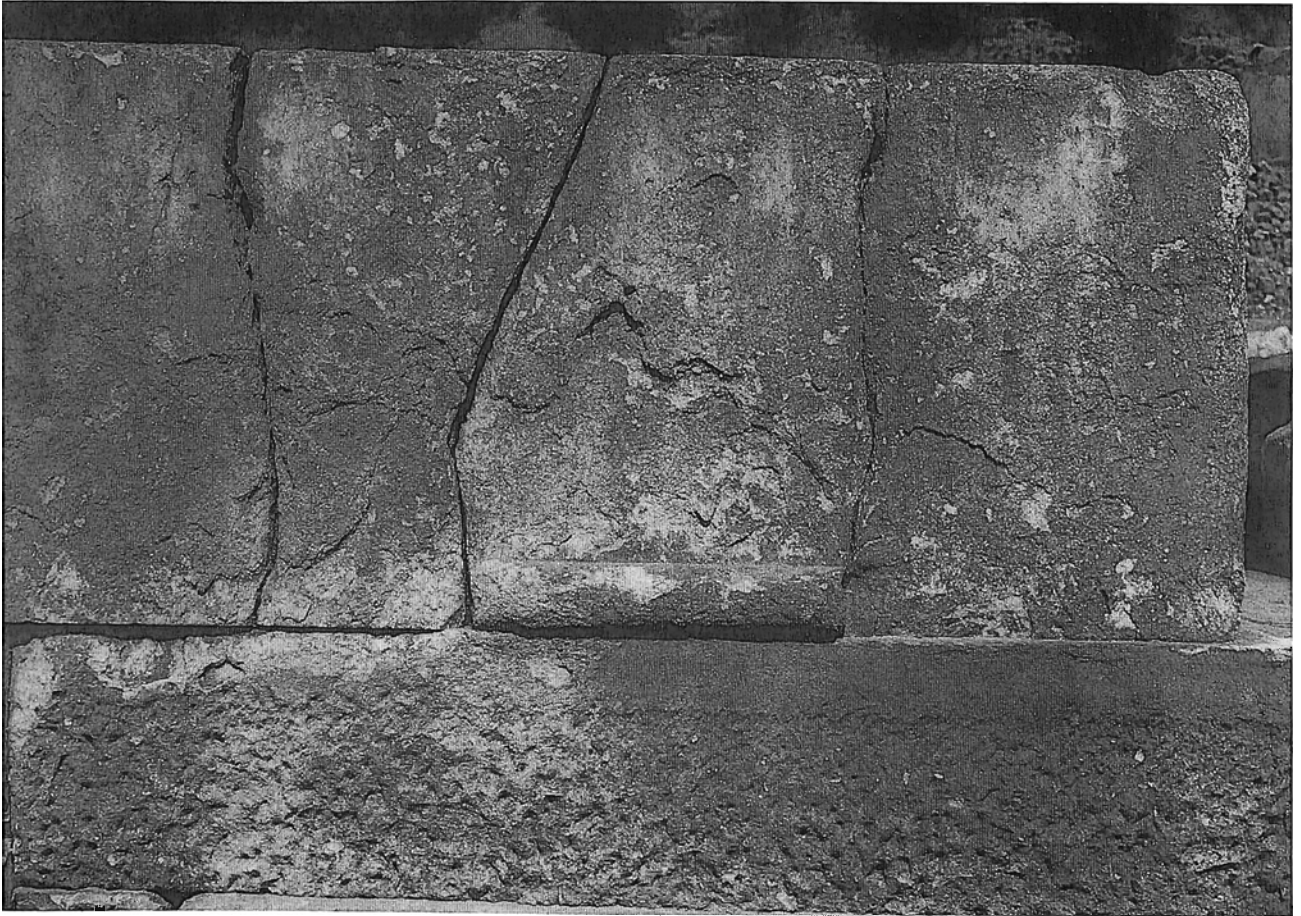
Pl.1-62 Deterioration of an orthostate block on the cross wall
