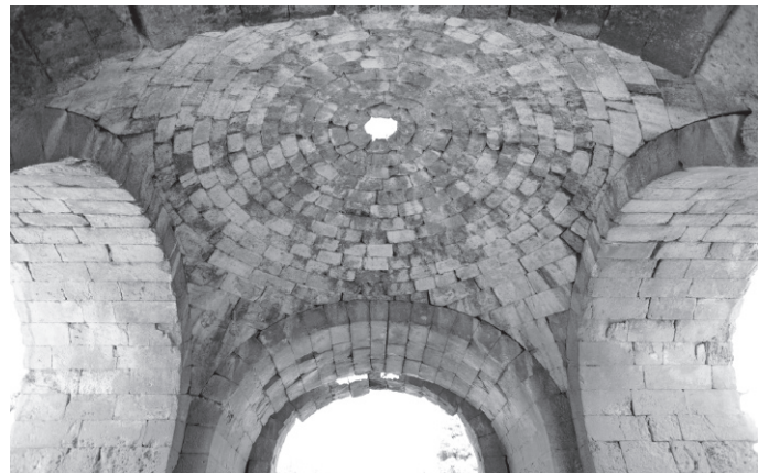
Fig. 17 Jerash, domical vault with pendentives of West Baths, looking from the south to the north
