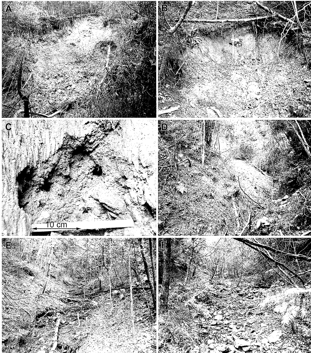
Fig. 5. Photographs of slope erosion and failures, and channels in the Sarukawa Experimental Watershed. (A) A channel sideslope failure (about 8 m wide) in the watershed 1. (B) A valley head collapse in the watershed 2. (C) Pipes formed on a collapse wall. (D) A slope failure at the headwater of the watershed 2. (E) A small channel having woody debris and sediment in the watershed 2. (F) The main stream of the watershed 2.
